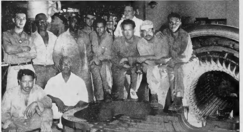
Shown above is a 75,000-kilowatt generating unit at No. 2 Powerhouse which is open for inspection by a group of employees under the direction of Ernest Ball, International General Electric representative. To the right is the armature of the generator, and in the foreground is part of the steam turbine. Mr. Ball will spend six or seven months in Aruba inspecting the various GE units in the refinery. In the group above are C. Jacob and C. Hughes, kneeling; standing from the left are A. Casali, J. Warren, R. Milan, H. Nixon, E. Maduro, R. Vanderlinden, Mr. Ball (behind Mr. Vanderlinden), G. Holsman, and A. Briezen.
